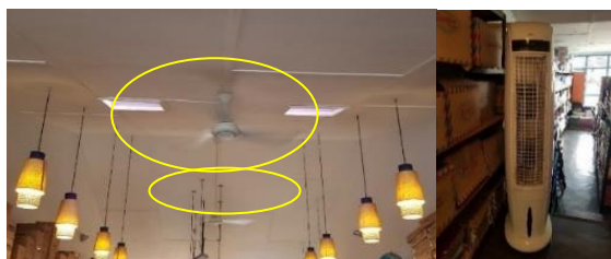
Figure 5. Ventilation at Nadhi Heritage
